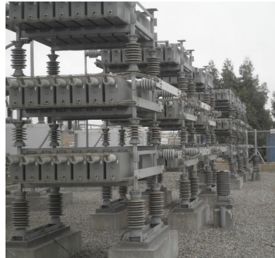
Figure 5 Filter capacitor banks.
