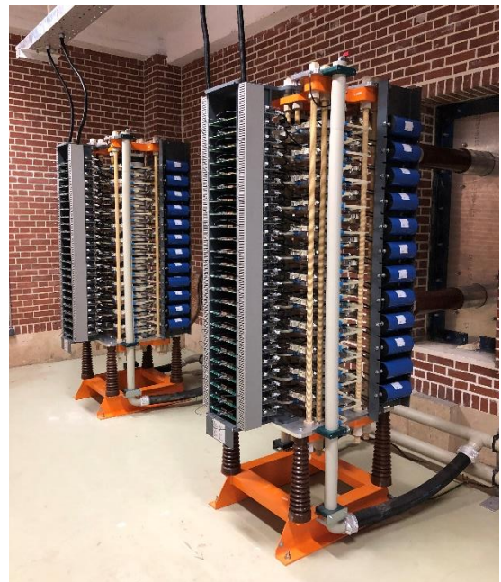
Figure 7 Medium voltage thyristor valves
