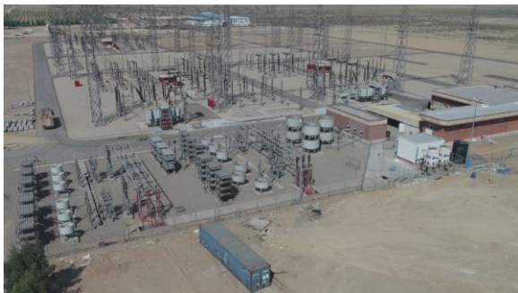
Figure 1 0 – 225 Mvar SVC system for EAF
