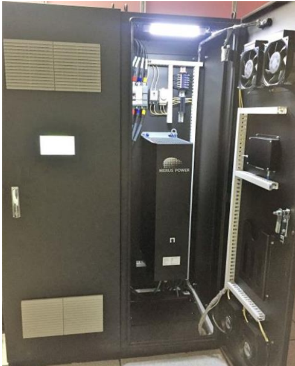
Figure 6 AHF 380V 60Hz 100A located at 2AHF-2A panel
