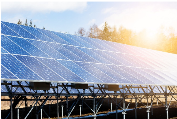
Figure 3 Solar power installation
